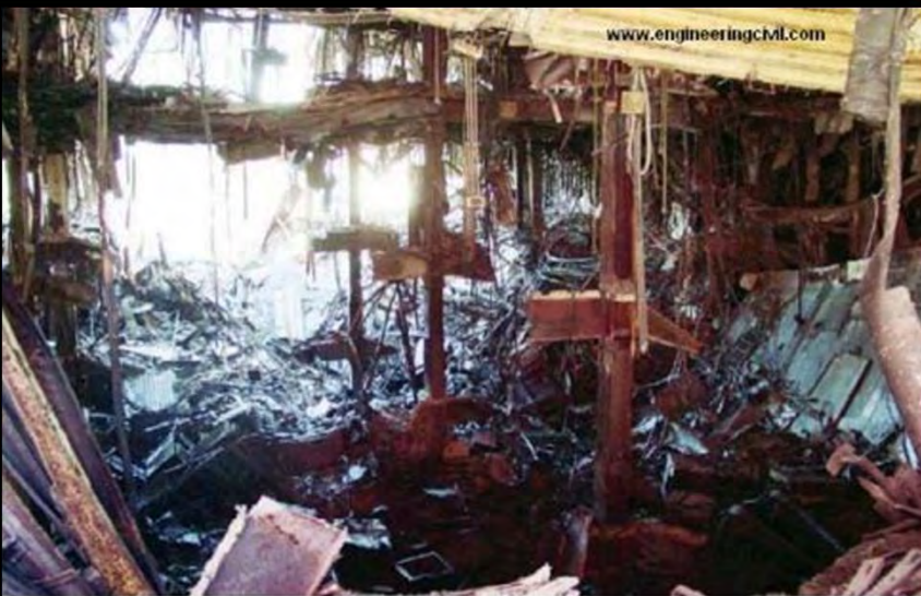
Figure 2. Internal Collapse Area in WTC 5 (World Trade..., 2002).
