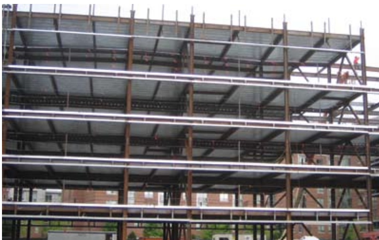
Consistent beam depths and non-regular column bays were key structural goals for NW35.
