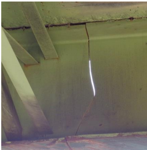
Figure 13: Full-depth Crack in Fascia Beam.
