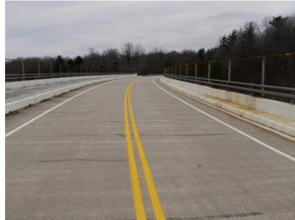
a) Before Rehabilitation
